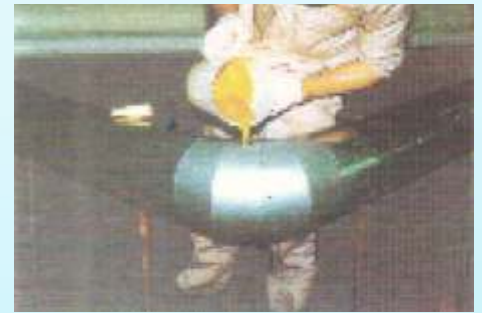
Pour Chemicals through opening
