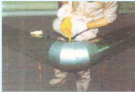
Pour Chemicals through opening
